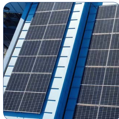
Roof-mounted Solar Photovoltaic Panels
